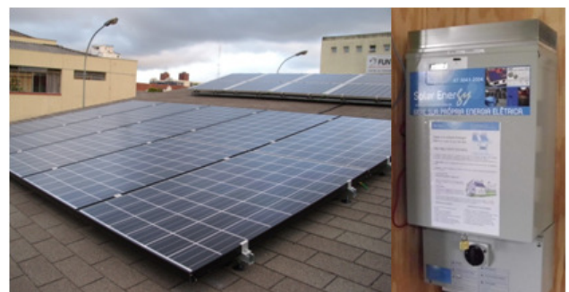
Figure 6 – Photovoltaic Panel and inverter of UTFPR, Curitiba. Source: [9].
